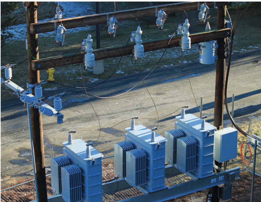
FIGURE 8.15 Three, single-phase MVPERs installed on a feeder. (© 2017 AMSC. All rights reserved.)
