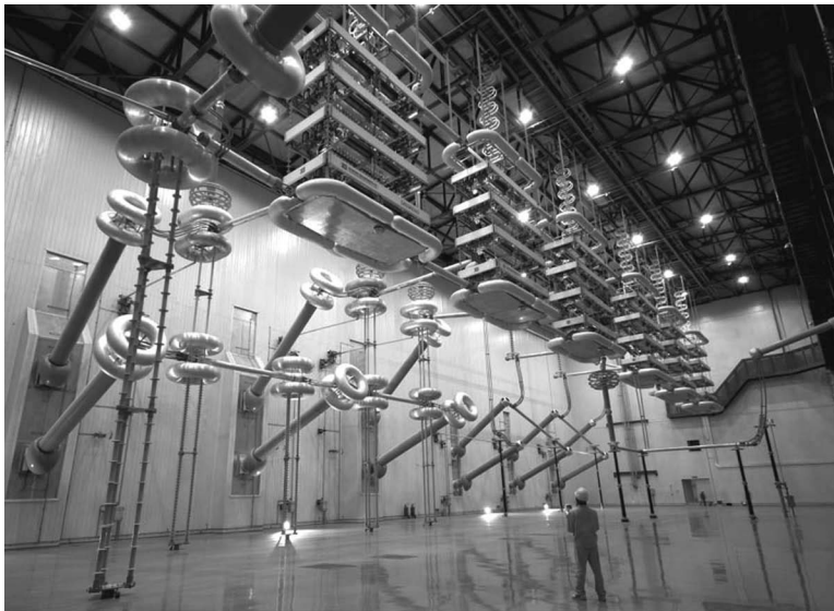
FIGURE 18.20 Conventional HVDC thyristor valve hall. (© 2012 Siemens. All rights reserved. With permission.)
