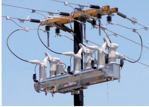
FIGURE 7.4 IntelliRupter® PulseCloser® fault interrupter. (© 2012 S&C Electric Company, Chicago, IL. All rights reserved.)
