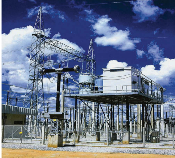
FIGURE 18.6 A series compensation installation. (© 2012 Siemens. All rights reserved. With permission.)
