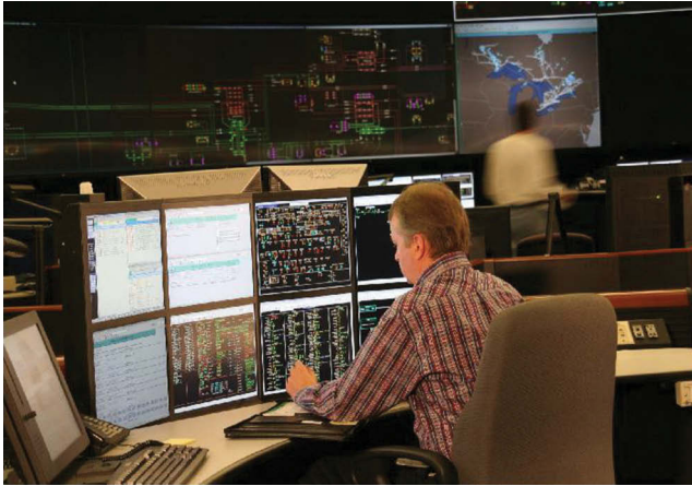
FIGURE 5.7 Control center operator console. (© 2016 General Electric. All rights reserved. With permission.)
