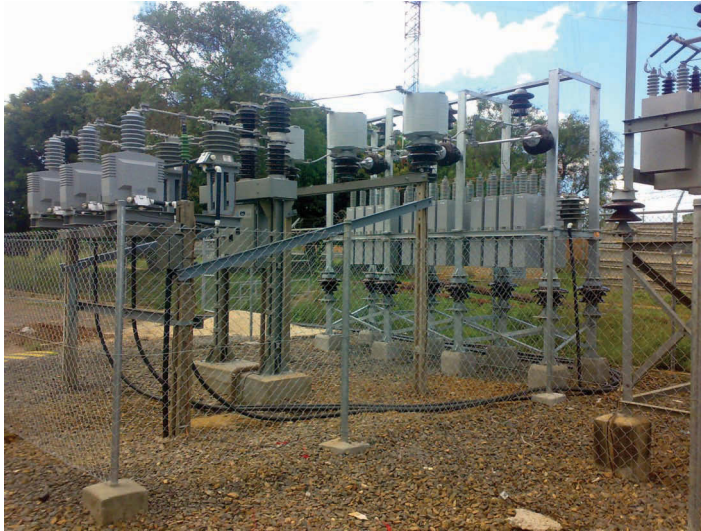
FIGURE 8.9 Photograph of a substation capacitor bank. (Courtesy of Siemens.)
