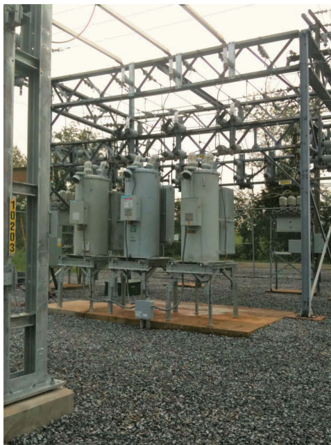
FIGURE 8.5 Photograph of three single-phase bus voltage regulators.
