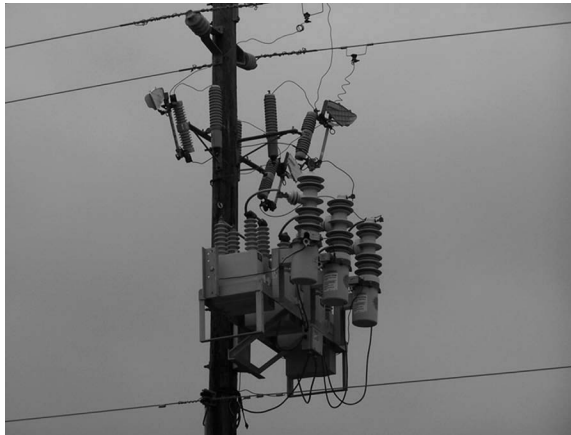
FIGURE 8.12 Photograph of a pole-top switched capacitor bank.
