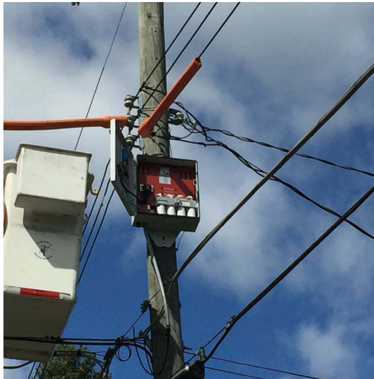
FIGURE 8.21 Secondary switched capacitor installed on a feeder. (© 2016 Gridco Systems. All rights reserved.)
