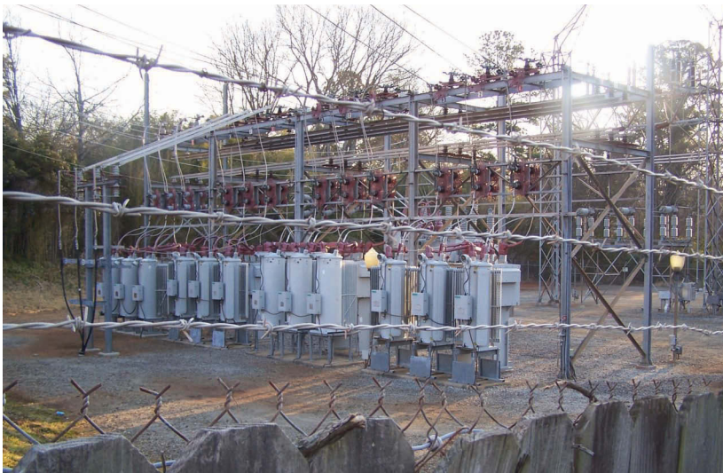
FIGURE 8.7 Photograph of single-phase voltage regulators on distribution feeders in the substation.
