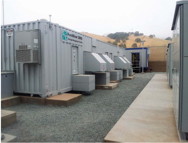
FIGURE 3.3 A 2-MW energy storage installed in a utility substation. (© 2016 S&C Electric Company. All rights reserved. With permission.)
