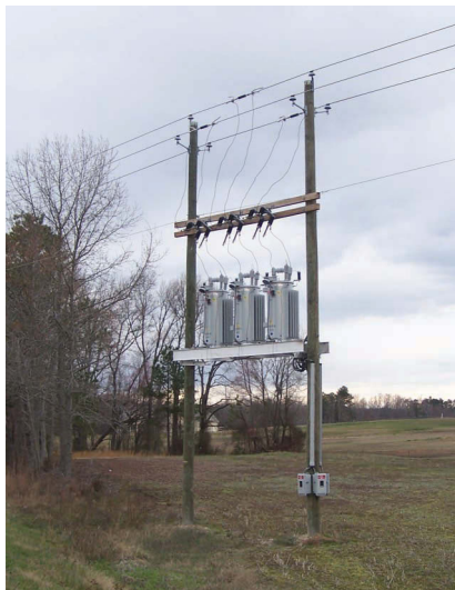
FIGURE 8.10 Photograph of three single-phase voltage regulators on a distribution feeder.
